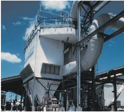
Dust collection system installed at Calcium Hypochloride manufacturing facility
