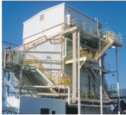
Wet electrostatic precipitator installed at fiberglass manufacturing plant
