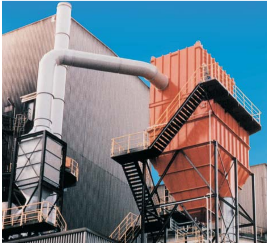
Dust collection system installed at anode paste plant
