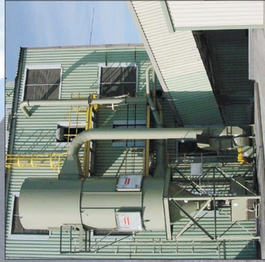
Filtration of crusher dust.
